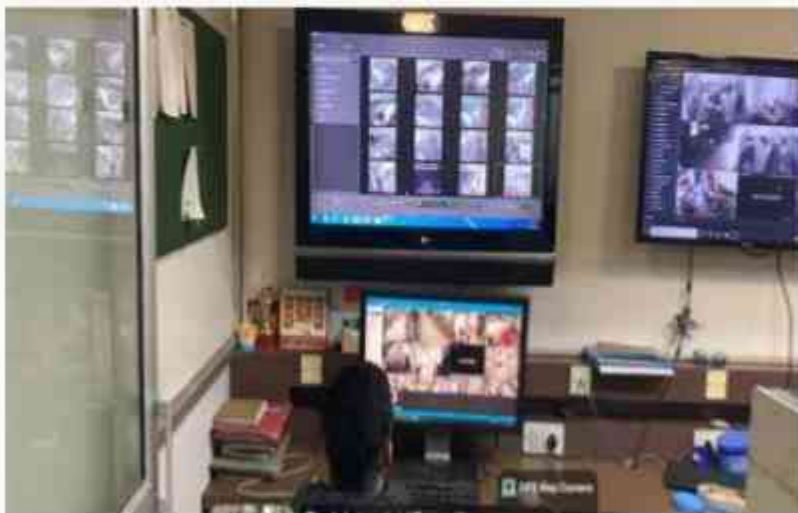
CCTV Surveillance Room
