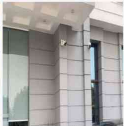
CCTV cameras outside buildings
